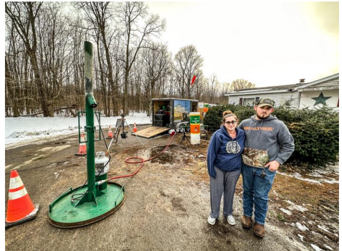
Residents of mobile home located 15' from the Bear Run #001 undocumented orphan well
